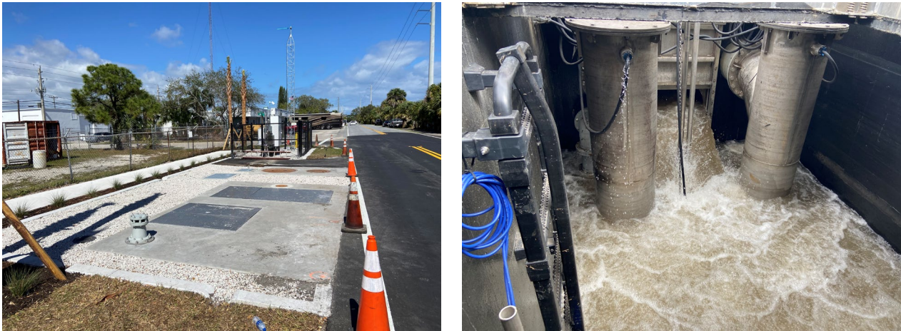
Figure 19: Juno Street Pump Station and Wet Well
