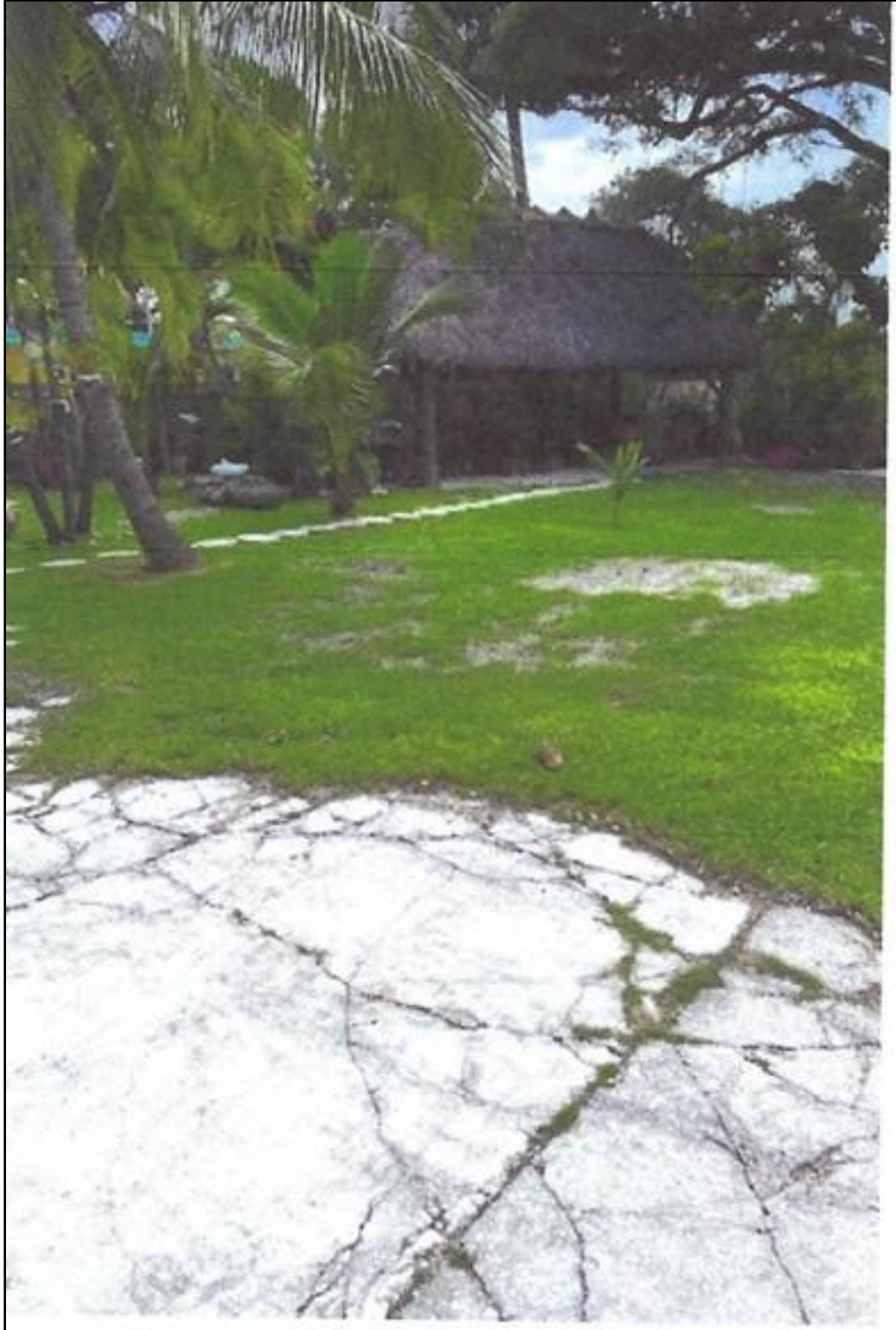
Figure 10. Project area overview of chickee hut and cement pads and walkways, facing southeast.
