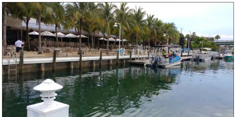
Figure 122 Image of needed seawall improvement.
