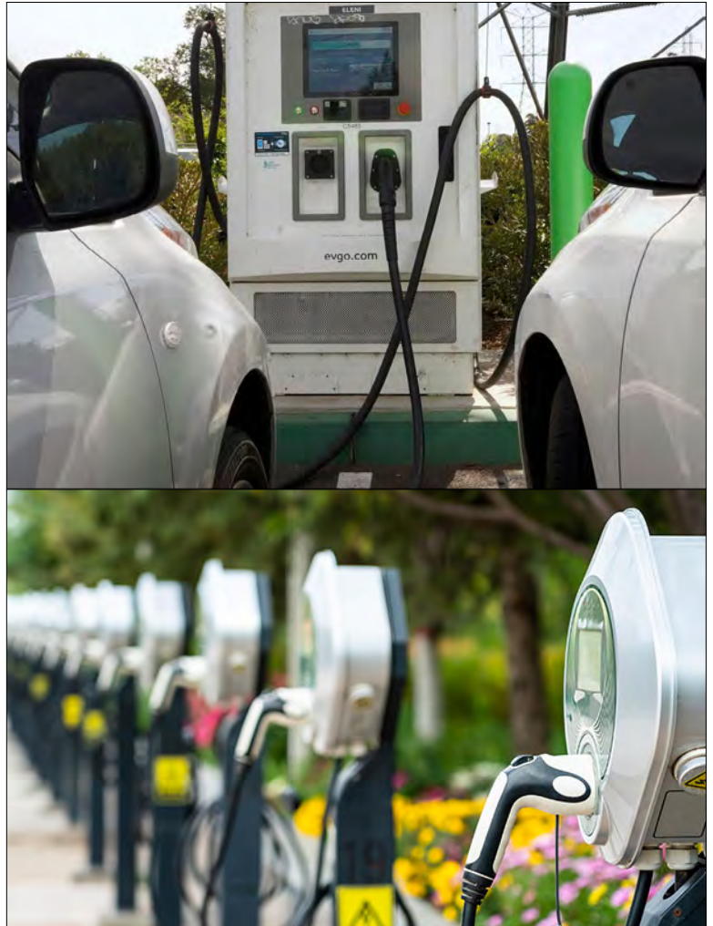
Figure 87 Examples above of electric vehicle charging infrastructure.
