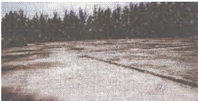
ABANDONED, UNSAFE PARKING
