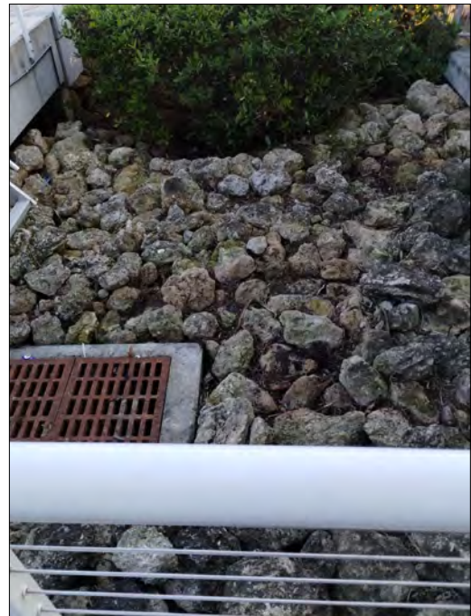
Figure 47 Stormwater outfall at Love Street
