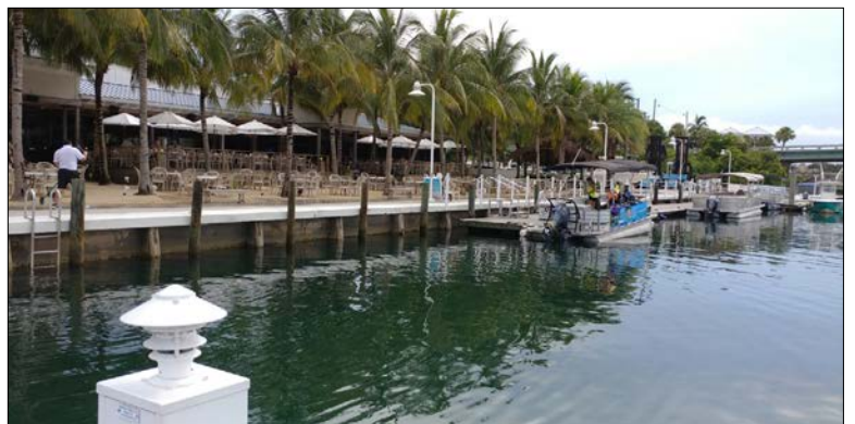
Figure 122 Image of needed seawall improvement.
