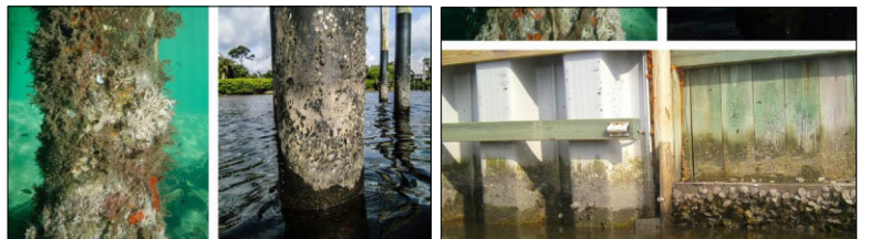
Figure 120 Pilings allow encrusting species to become established.
