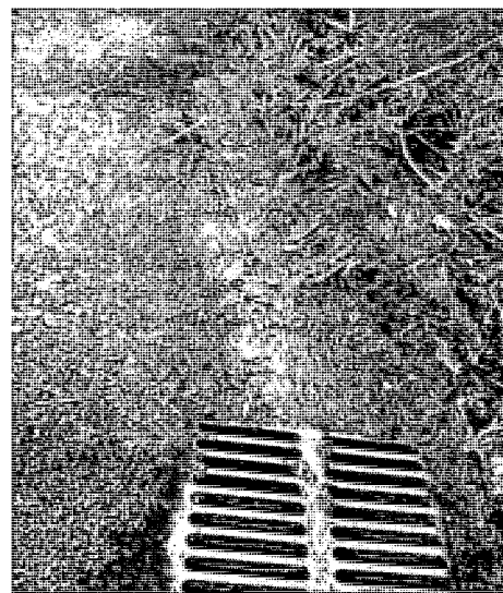
Wash-out of gravel and other debris into drain grate.
