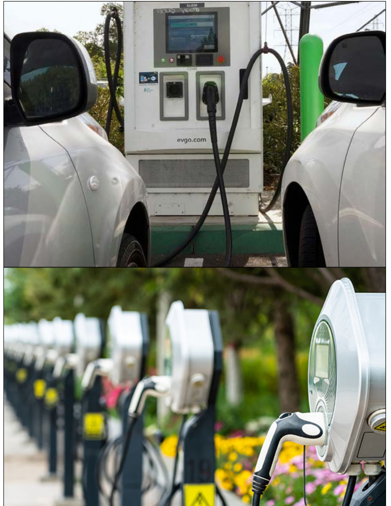
Figure 87 Examples above of electric vehicle charging infrastructure.
