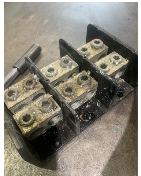
Connection block corroded from water intrusion
